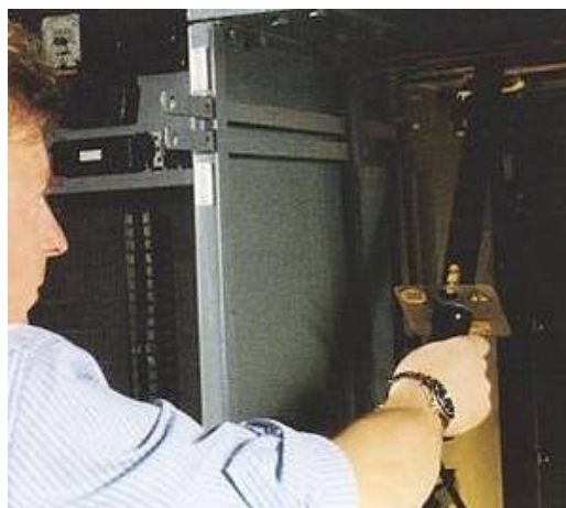
HVI - Switchgear Testing
